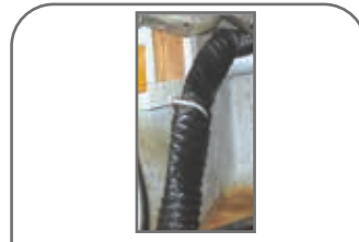
Crushed vent ducting, will impede proper and safe venting of fumes. Replace damaged duct
